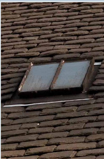
A traditional iron rooflight set into a West Highland slate roof. The small size, low profile and 'portrait' format are typical characteristics. © N. Haynes.
